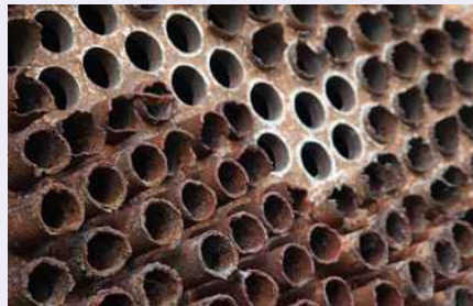
Corrosion in Boiler Tubes
